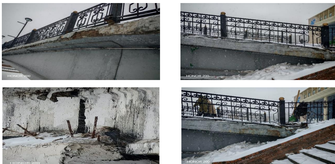
Figure 4. Reinforced concrete support of a road bridge on K. Satpayev Street (Astana) affected by corrosion (author's work)
