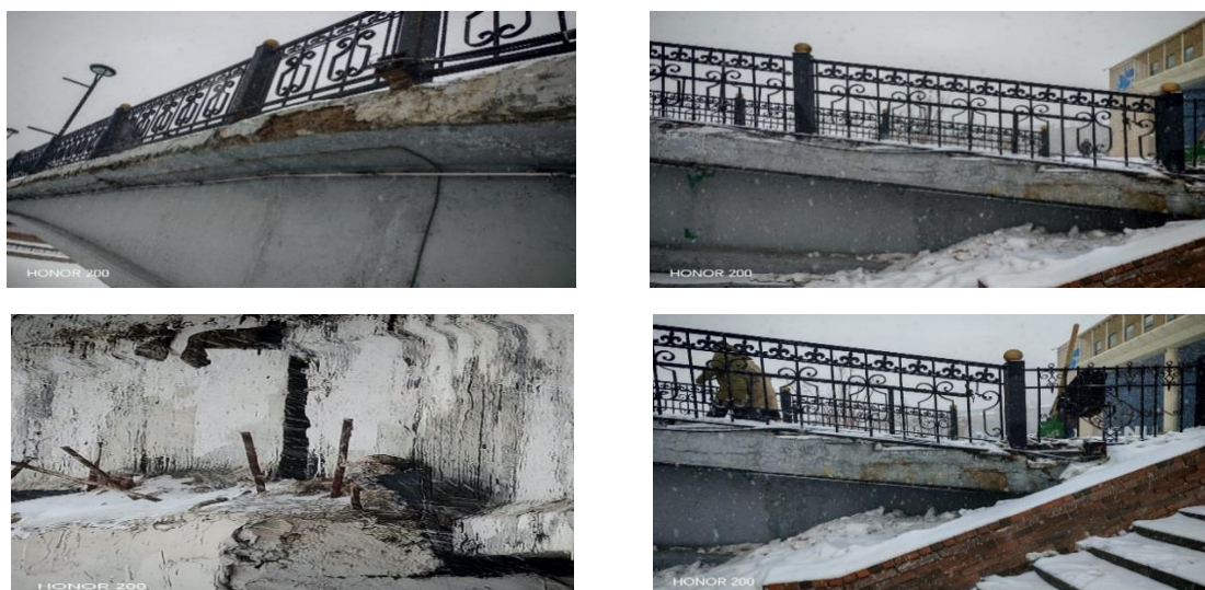
Figure 4. Reinforced concrete support of a road bridge on K. Satpayev Street (Astana) affected by corrosion (author's work)
